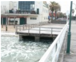
Kerferd Road Pier Port Melbourne March 2003 drain 004
